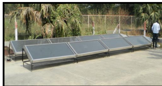
Plate 2: Solar collector (8 Nos.)
