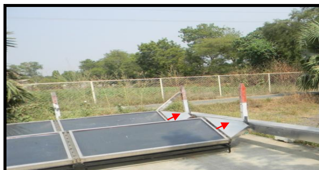
Port 1 & 2 between solar collector row and main duct
